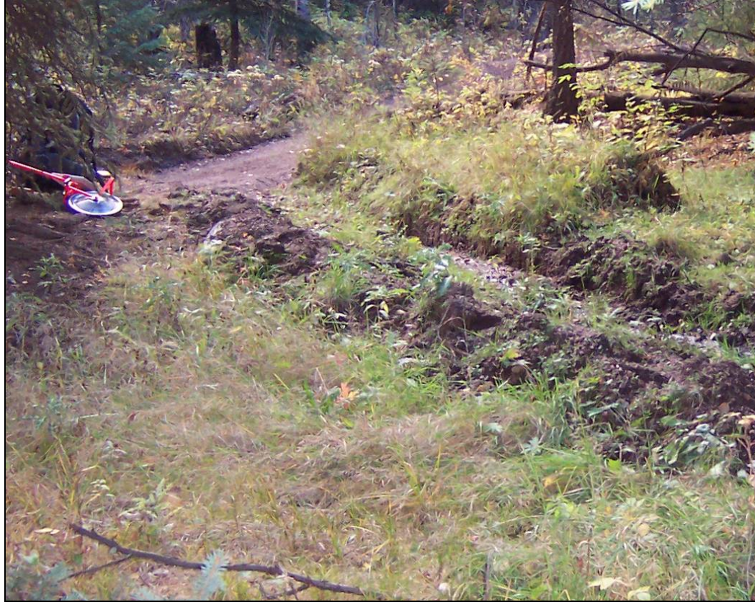
Figure 3.6. A pushout drainage channeling runoff from the Devil's Slide trail directly into a perennial stream channel that is just off the right side of the photograph.
