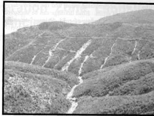
Figure 3. Road-induced debris flows in northwest Washington state, USA. The debris flows initiated in the colluvial hollows on the upper road were triggered by road runoff, and these triggered the failures at the road-stream crossings on the lower road. The road was built prior to the implementation of best management practices and large fill volumes were placed within colluvial hollow and inner gorge landforms.
