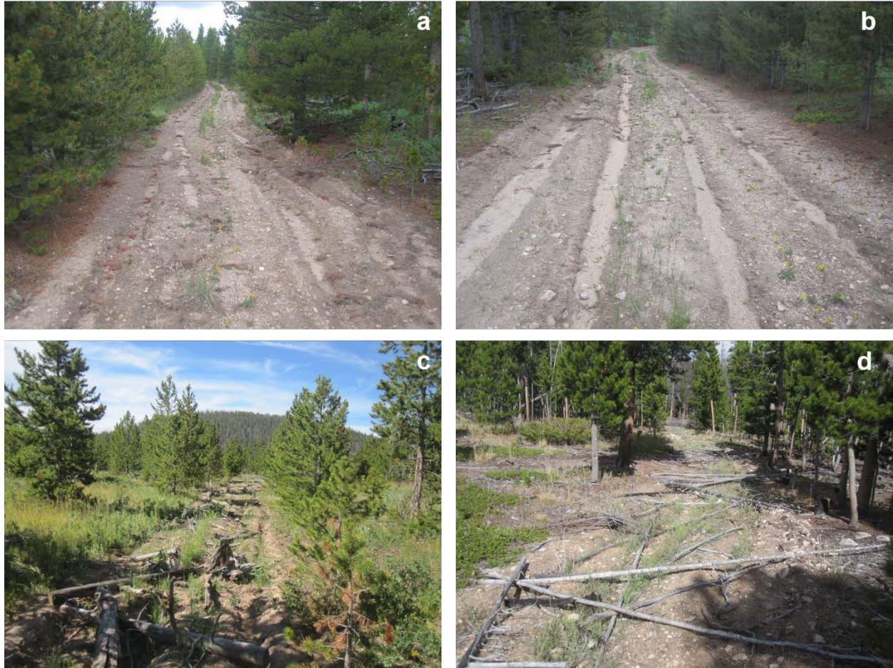
Figure 3.8. Typical road segments one year after decommissioning. a) Segment with 4% slope that was only ripped. The road surface shows evidence of erosion, but all of the eroded sediment was trapped in the furrows created by the ripping. b) Segment with 9% slope that was only ripped, showing much more eroded, transported, and deposited sediment. c) and d) Road segments that were ripped and mulched showing much less erosion due to the mulch plus greater vegetative regrowth and slash cover compared to the segments that were only ripped.
