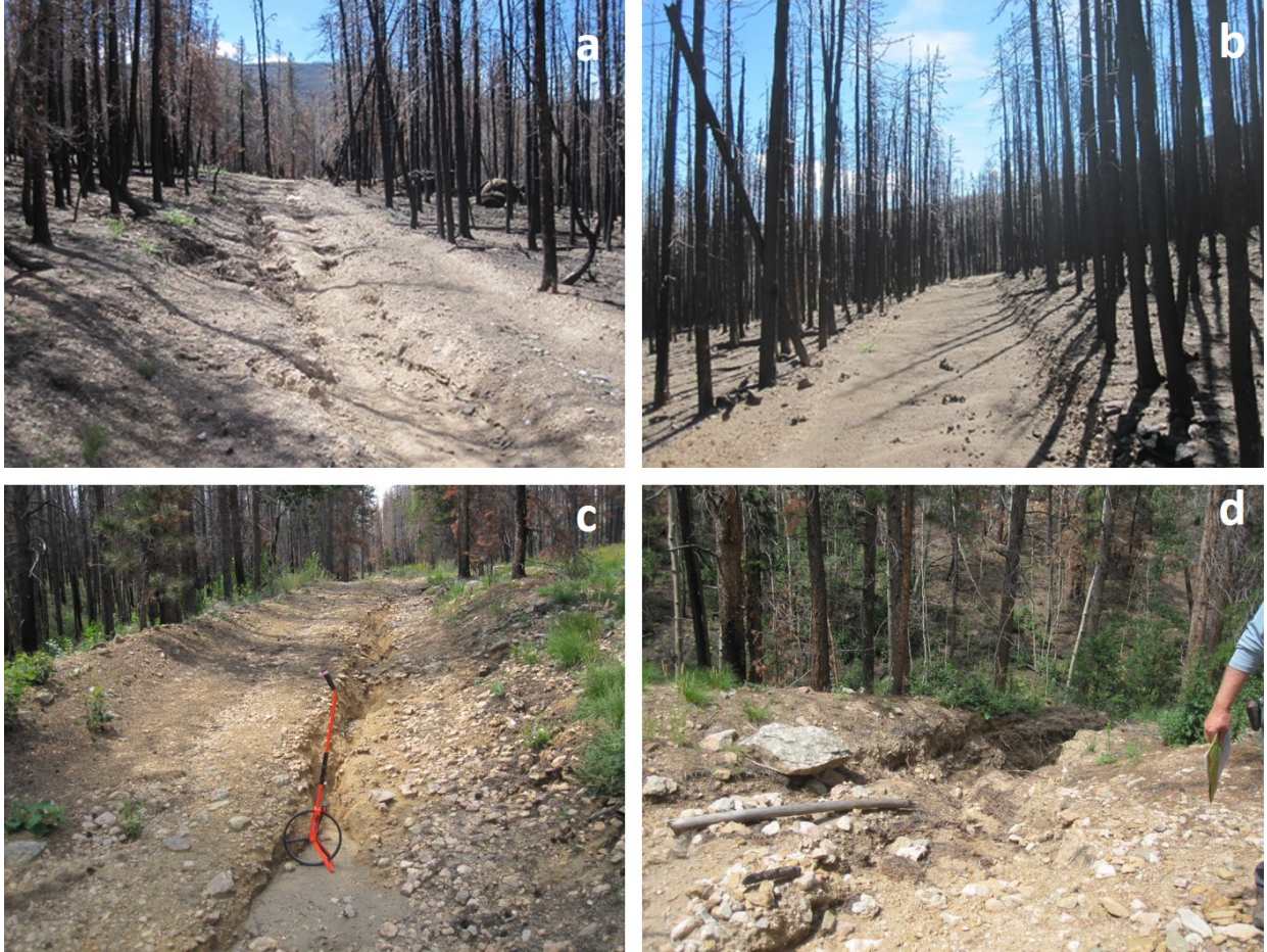
Figure 1.4. Representative road segments along Old Flowers Road. a) Road segment with 10% slope and road surface rilling below an area that burned at high severity. b) Road segment with only 2% slope below an area burned at high severity with no rills due to deposited sediment. c) Road segment below an area that burned at moderate severity showing how the one rill in the wheel track closest to the upper side of the road captures all of the runoff from the burned hillslope above the road. d) Single, deeply incised gully leaving a 51-m long road segment that was in an area that burned at high severity. This gully extended at least 10 m to the ephemeral stream at the base of the slope, and the large size of this drainage feature can be attributed primarily to the combination of runoff from the burned hillslope and the 15% slope of the road segment.
