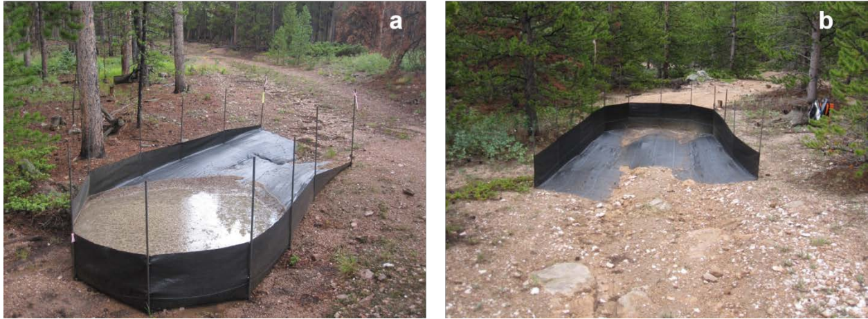
Figure 3.2. Sediment fence at a drainage outlet (a) and on the road surface (b).
