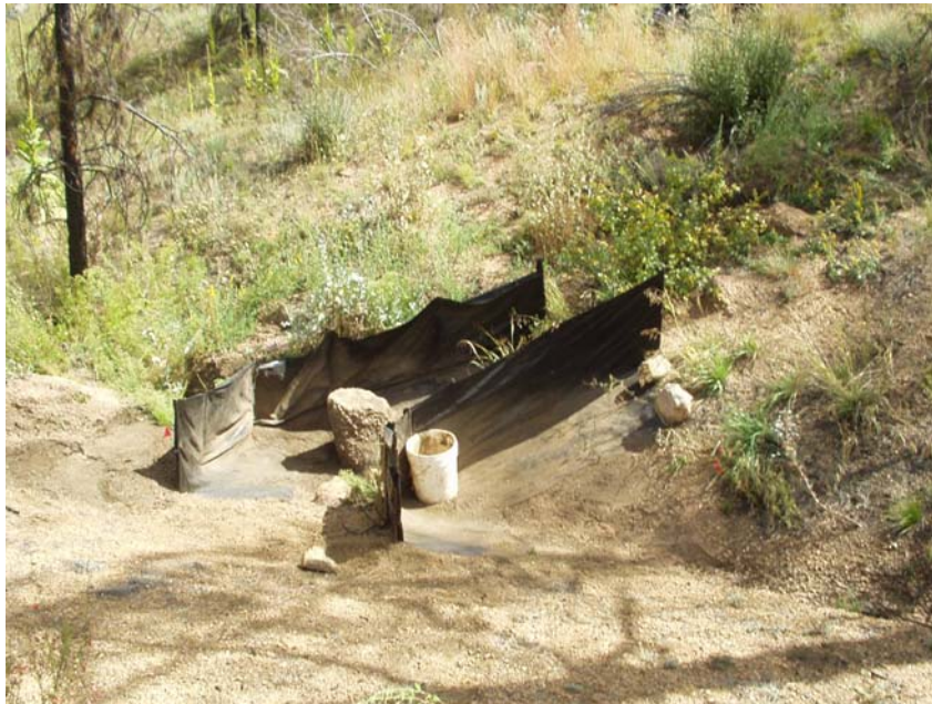
Figure 2. Two sediment fences in a swale in the Hayman fire. The lower fence is designed to capture any sediment that spills over the upper fence. Total storage capacity is about 2 Mg of wet sediment. The 20-L bucket in the upper fence is on the fabric apron laid in front of each fence.
