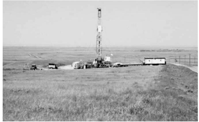
A new oil well being drilled in prime endangered sage-grouse habitat in southeastern Alberta. Photo by Cameron L. Aldridge.
